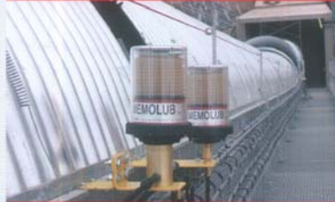
Conveyor lubrication in a quarry
